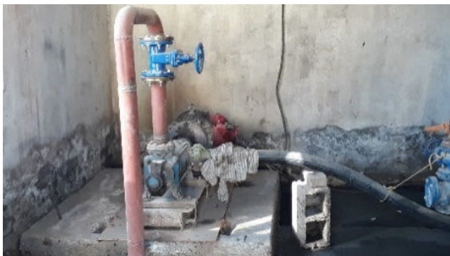
Figure 3. Pump station(after filtering) pump water for landscaping).
